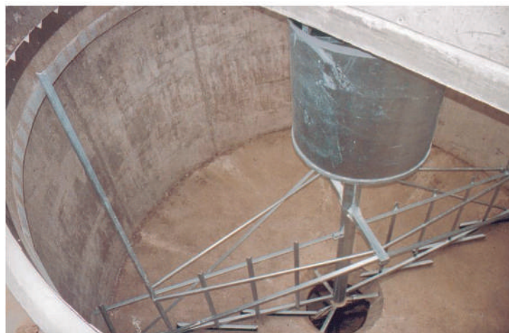
Gravity sludge thickener PACIFIC
